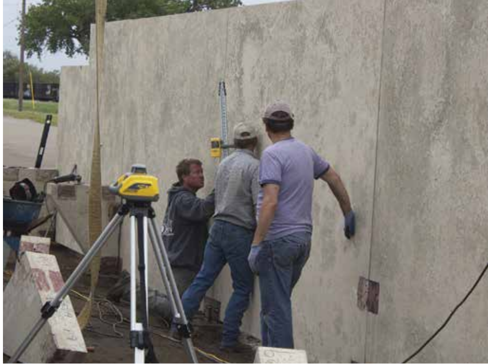
Students designed and constructed a six-panel precast concrete monument along the banks of the Missouri River in Mobridge, S.D., to serve as the focal point for a gathering spot.
